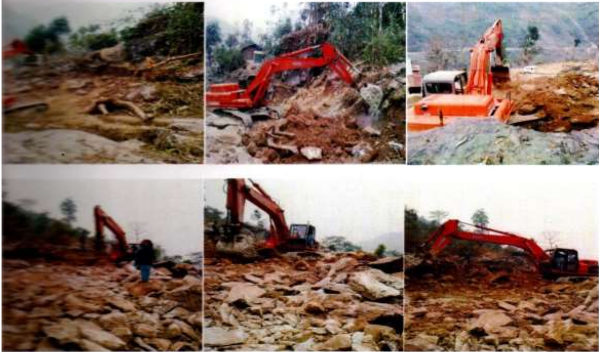
Leveling work in progress at Rehip, Tokal Bermiok, South Sikkim for construction of Composite Rehabilitation Centre.
